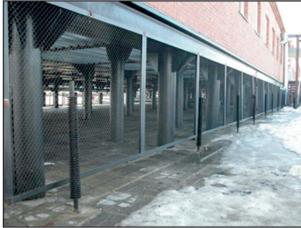
Fig. 9. Vertical cooling systems at Yubileinoe field
