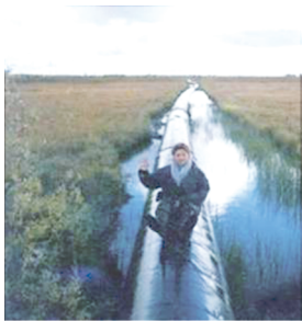
Fig. 6. Pipeline flooded as a result of ground ice thawing (photo by Ya. Panova)
