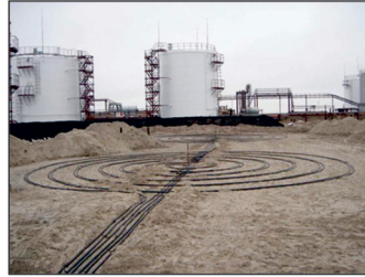
Fig. 10. Horizontal cooling systems at base of tanks
