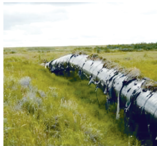
Fig. 7. Emergence of a pipeline and soil subsidence beneath it
